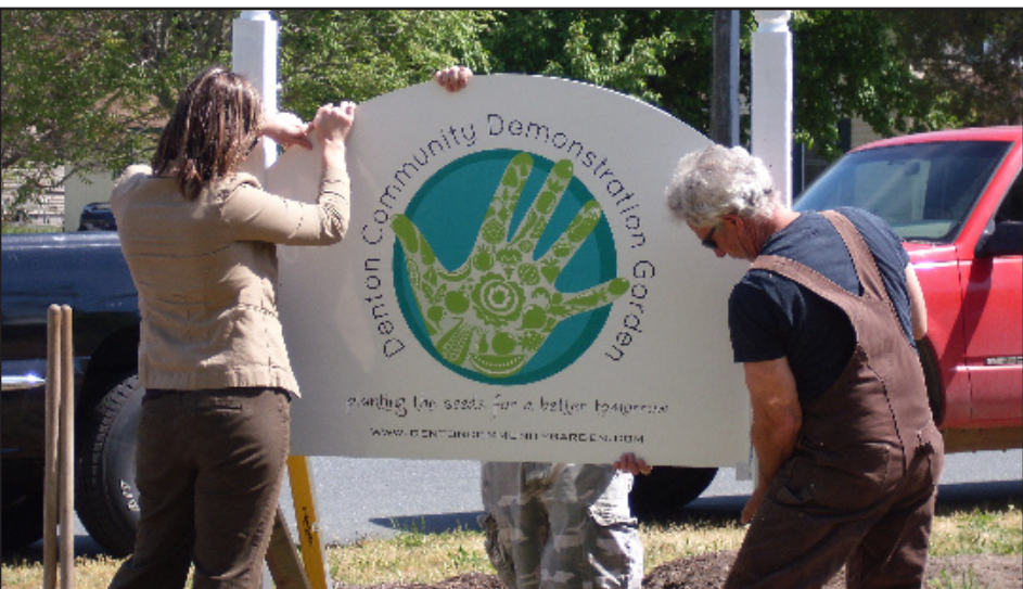
Volunteers Christina Lippincott and Mickey McCrea install a sign for the Community Demonstration Garden next to the Fourth Street Parking Lot.
